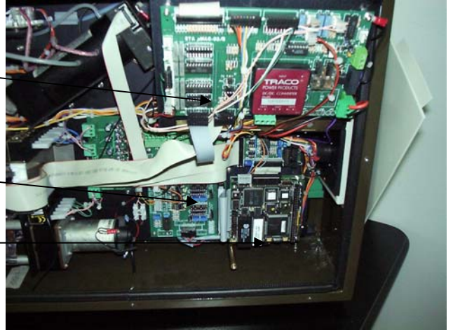
right side internal electronic compartment
